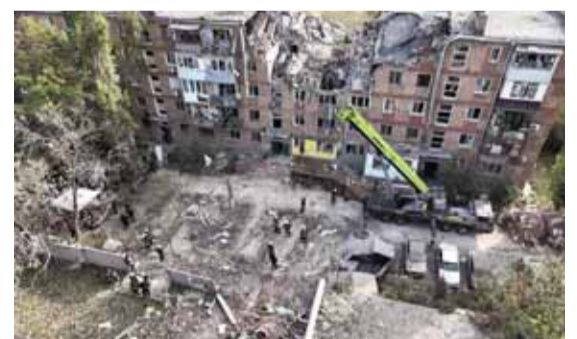
MYKOLAIV: Photo shows damage to a residential building after a strike in Mykolaiv, amid the Russian invasion of Ukraine. — AFP
