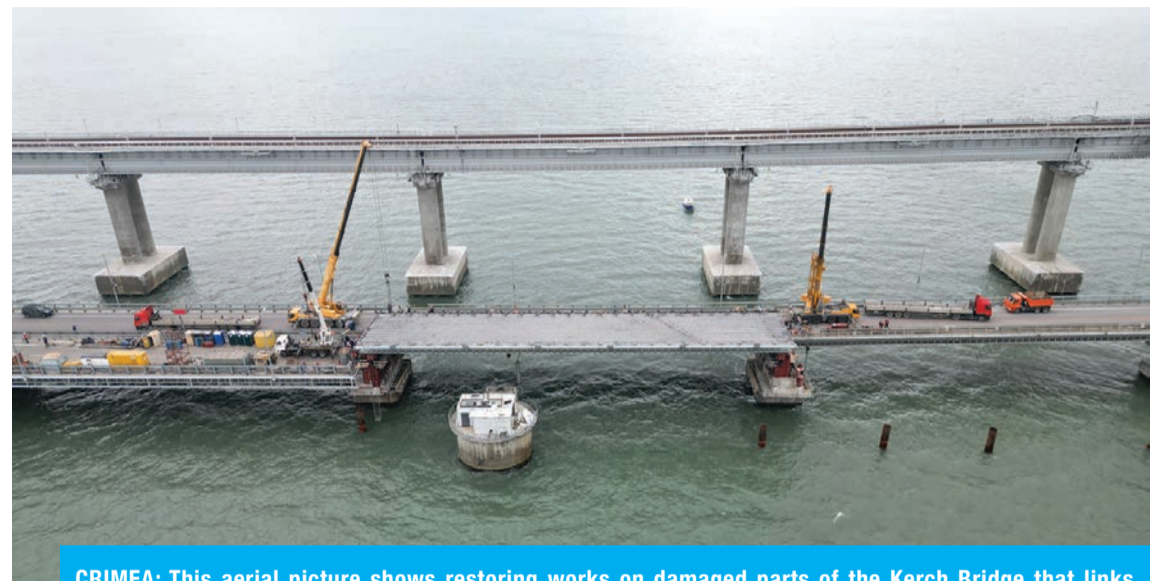
CRIMEA: This aerial picture shows restoring works on damaged parts of the Kerch Bridge that links Crimea to Russia, which was hit by a blast. —AFP
