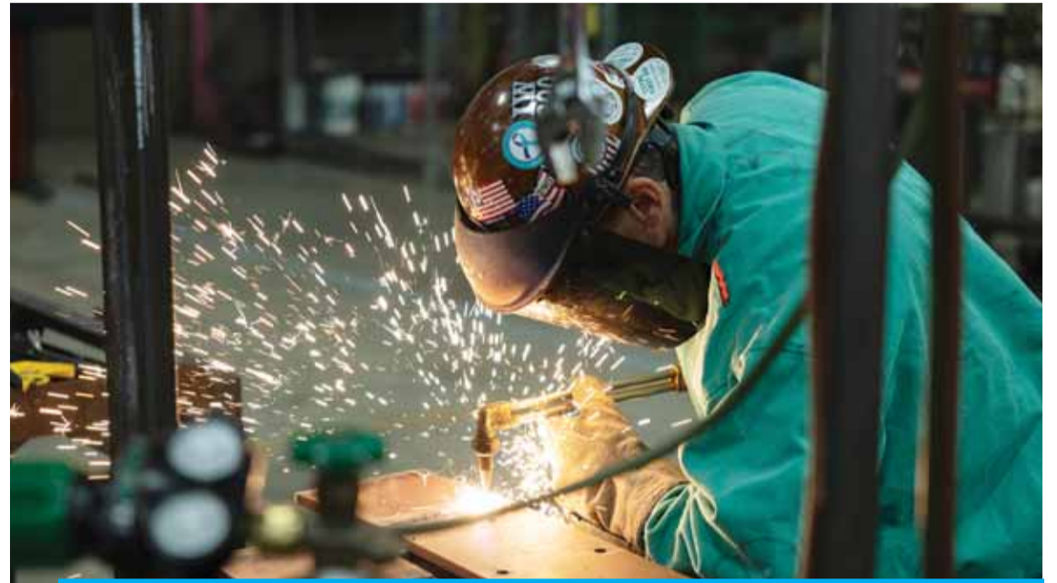
DAYTON, US: Matthew Atha, a 54-year-old apprentice, does steel work at Ironworkers local 29 during an apprenticeship in Dayton, Ohio. —AFP
