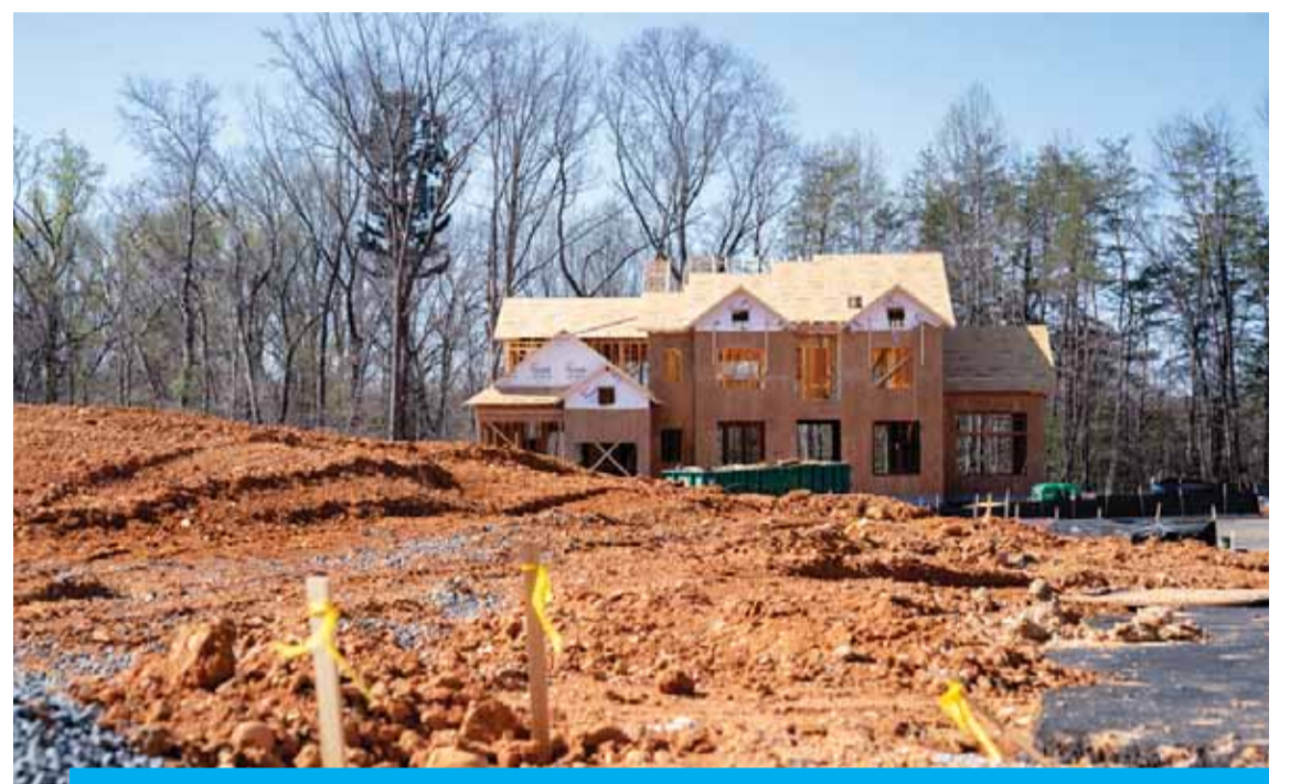
FALLS CHURCH, US: In this file photo, a home under construction in a new housing development in Falls Church, Virginia. US new home sales plunged 16.6 percent in April, even as prices continued to climb, according to government data released on May 24, 2022. —AFP
