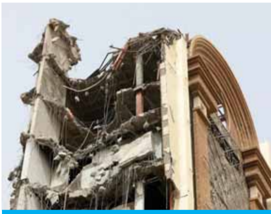
ABADAN, Iran: A picture shows a view of a collapsed ten-storey building, as rescue operations continue in the southwestern city of Abadan on May 24, 2022. —AFP
