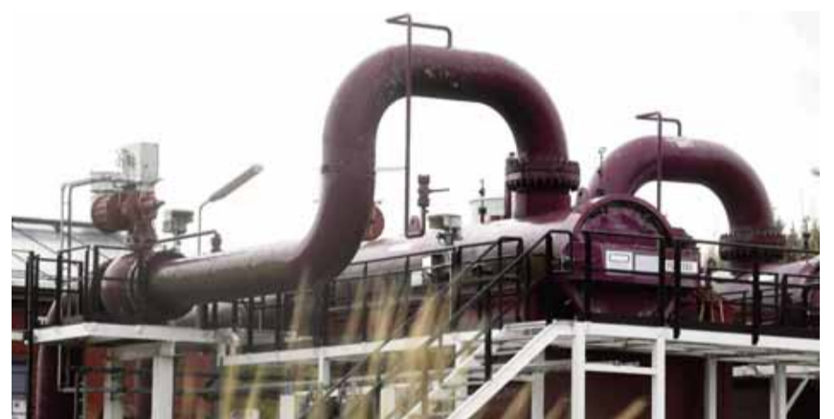
IMATRA, Finland: In this file photo taken on May 12, 2022 pipes at the Gasum plant are pictured in Raikkola, Imatra, Finland. Russia on May 20 stopped providing natural gas to neighboring Finland, which has angered Moscow by applying for NATO membership, after the Nordic country refused to pay supplier Gazprom in rubles. — AFP
