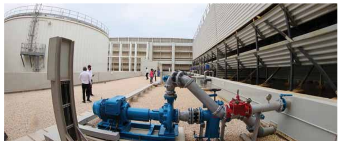
DOHA: A picture shows parts of the cooling system at the Al Janoub Stadium.
