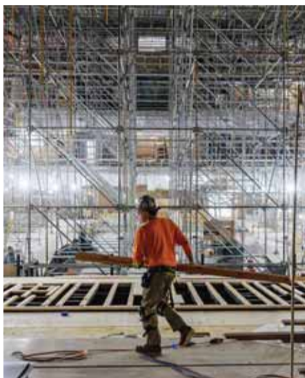
Construction workers build the stage during a press tour of the newly revitalized David Geffen Hall in New York City.
