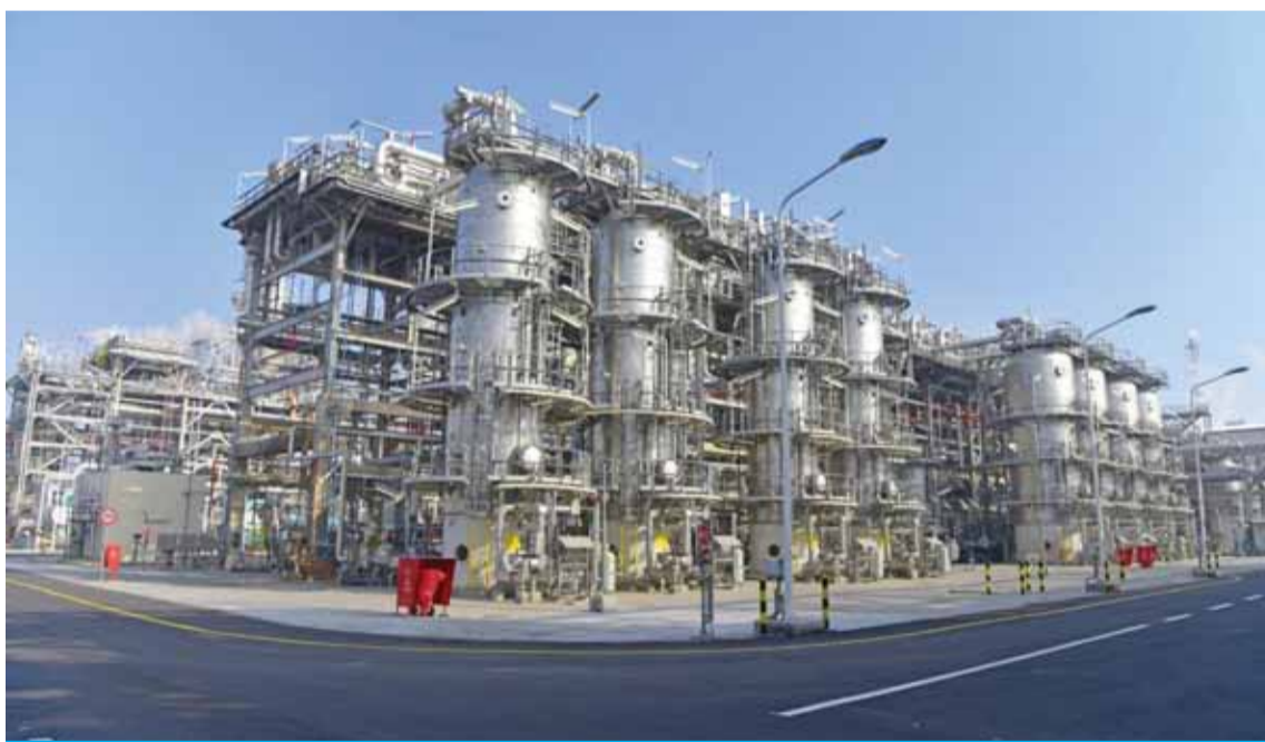
KUWAIT: The fifth liquefied gas line at Mina Al-Ahmadi Refinery. — KUNA
