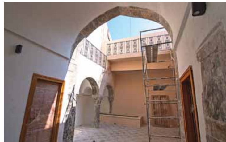
A picture shows a view of a traditional house during reconstruction work.
