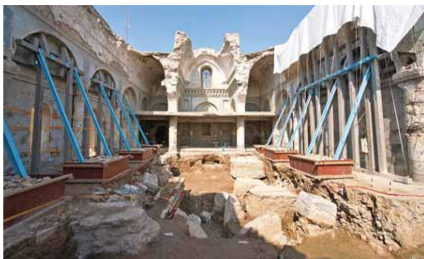
A picture shows a view of renovations at the Church of the Immaculate Conception (Al-Tahira-I-Kubra) supported by the United Nations Educational, Scientific and Cultural Organization UNESCO, in the old town of Iraq's northern city of Mosul. — AFP photos
