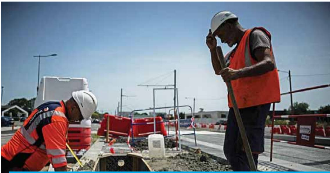
GIRONDE, France: Men are at work at a construction site in Merignac, outside Bordeaux, southwestern France, on June 14, 2022 as a heatwave hits France. France's weather service said a heatwave would hit southern regions from late June 14, worsening a drought across much of the country that is threatening farm harvests. — AFP
