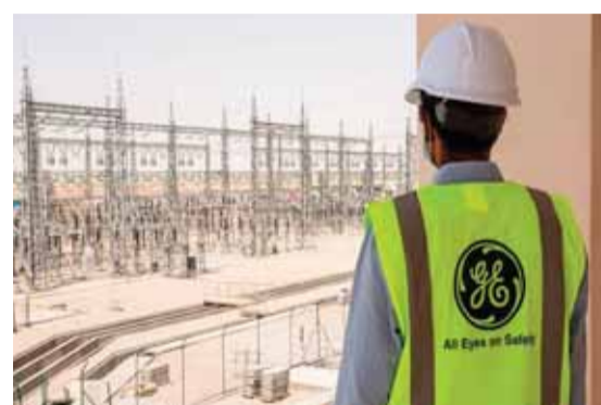
NASIRIYAH: A General Electric employee stands near a power plant in Nasiriyah, Iraq.—AFP
