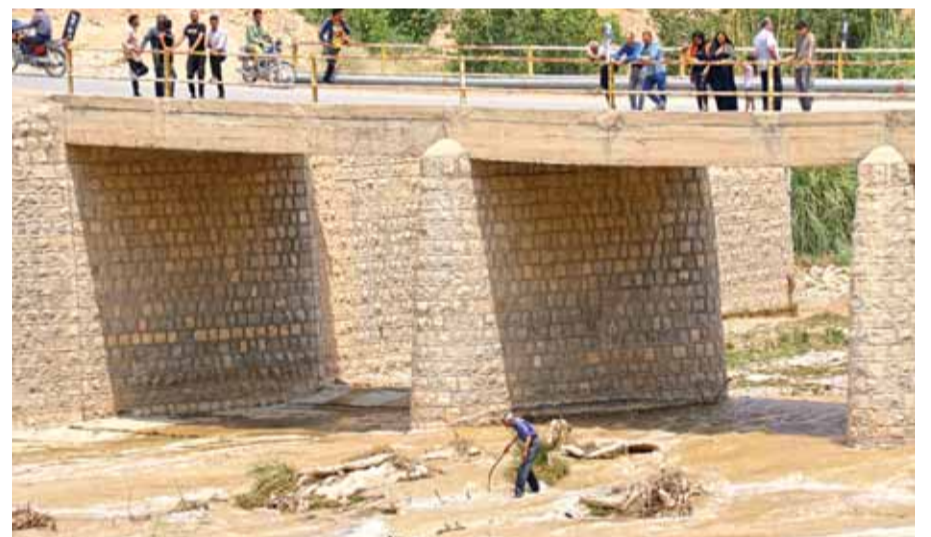
ESTAHBAN: People stand on a bridge above a river, after flooding caused by heavy rainfall in southern Iran's Estahban county, that reportedly killed at least 21 people. — AFP
