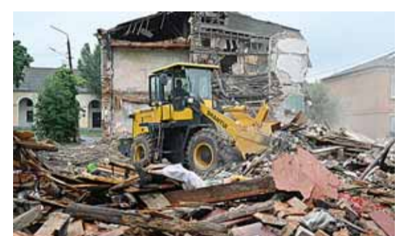
CHUGUIV, Ukraine: A Ukrainian rescue worker removes debris with a bulldozer from a damaged building partially destroyed after a shelling in the city of Chuguiv, east of Kharkiv. —AFP
