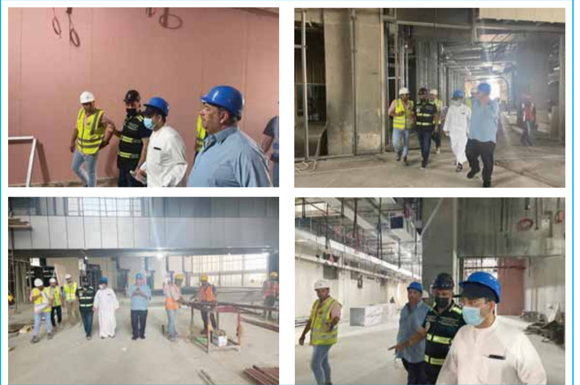
KUWAIT: Health Ministry Undersecretary Dr Mustafa Redha inspected the project of the new Kuwait Cancer Fighting Center in Sabah Specialized Medical zone. The project covers 65,000 square meters. The new building will be 22,4762 square meters with a 618-bed capacity.
