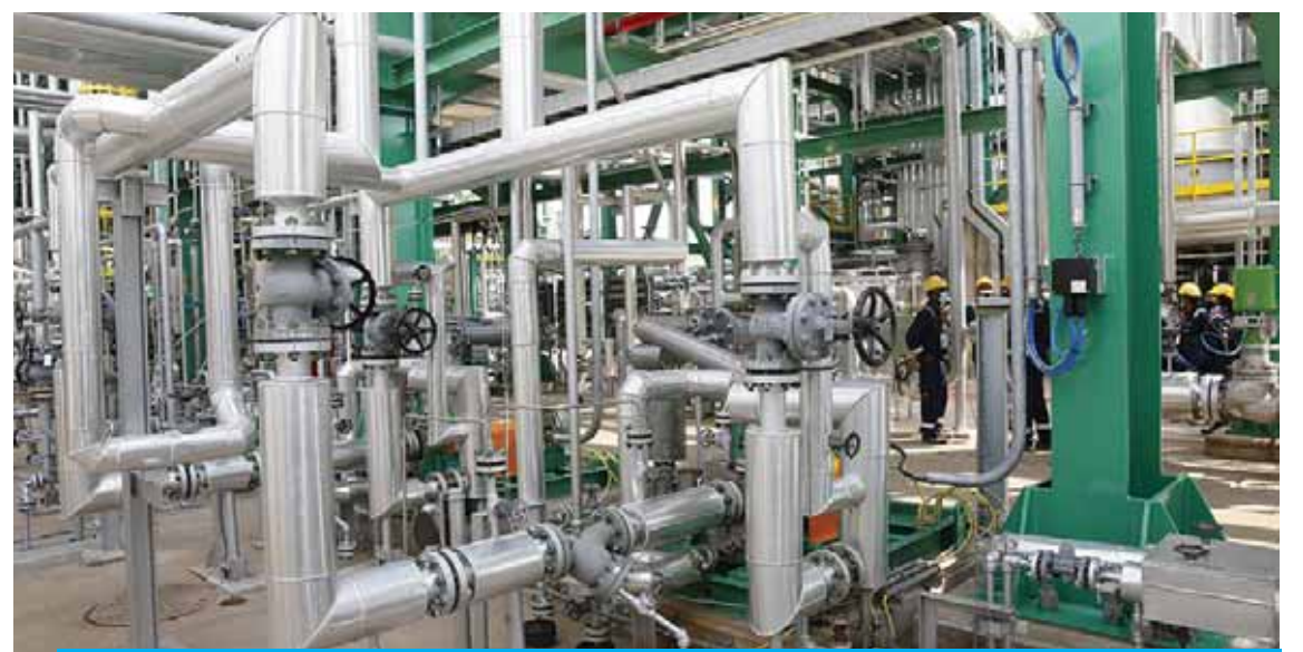
LUANDA: A general view of the refinery at the state oil company, Sonangol, in Luanda. Oil-rich Angola on Thursday unveiled a new production unit that will increase fourfold the output at its sole refinery as it seeks to reduce dependency on fuel imports.— AFP
