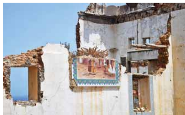
A damaged building in the Casbah of Algiers.—AFP photos
