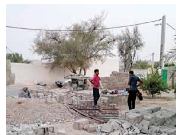
SAYEH KHOSH, Iran: A view of destruction in the aftermath of an earthquake in this village in Iran's southern Hormozgan province. — AFP
