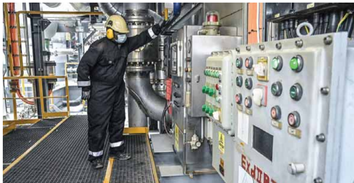
KIBUYE, Rwanda: Cyprien Bigirimana, a maintenance technician, seen inside the barge extracting methane gas on Lake Kivu, at the KivuWatt power plant in Kibuye, Karongi District, in the Western Province of Rwanda. — AFP
