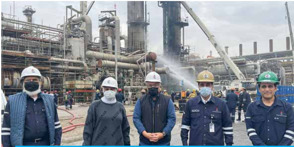
KUWAIT: A handout picture provided by KNPC on Friday shows Oil Minister Mohammad Al-Fares with KNPC officials at Mina Al-Ahmadi refinery as firefighting personnel extinguish a fire which broke out during maintenance work. — AFP
