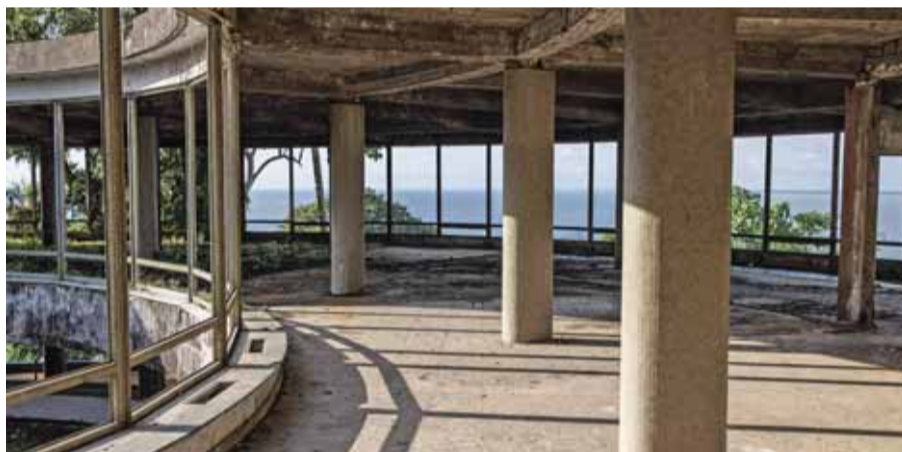
An old lounge area is pictured in the dilapidated Ducor hotel in Monrovia.
