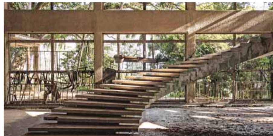
An old stairway is pictured in the dilapidated Ducor hotel in Monrovia.
