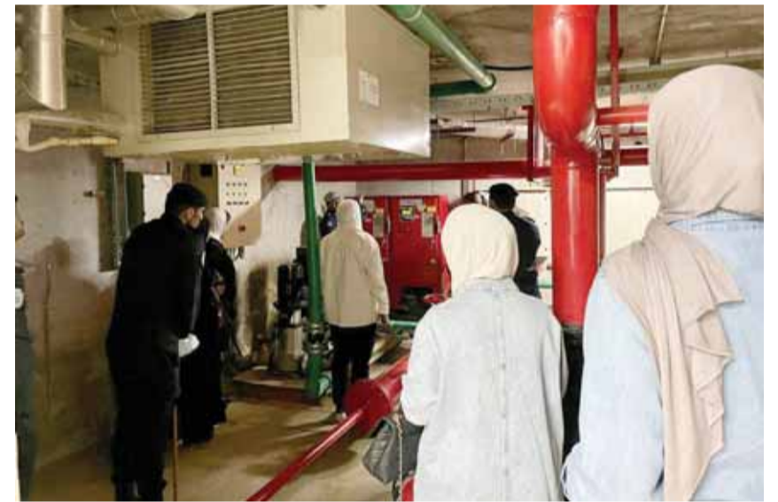
The program was conducted in order to familiarize the participants with the mechanisms of firefighting equipment, fire alarms and other engineering services.
