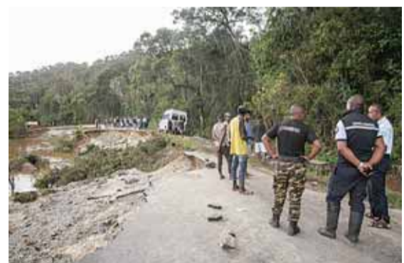
RANOMAFANA, Madagascar: Residents look at the partially collapsed RN25 road in Ranomafana yesterday following the passage of cyclone Batsirai. Cyclone Batsirai swept out of Madagascar yesterday after killing 20 people. —AFP
