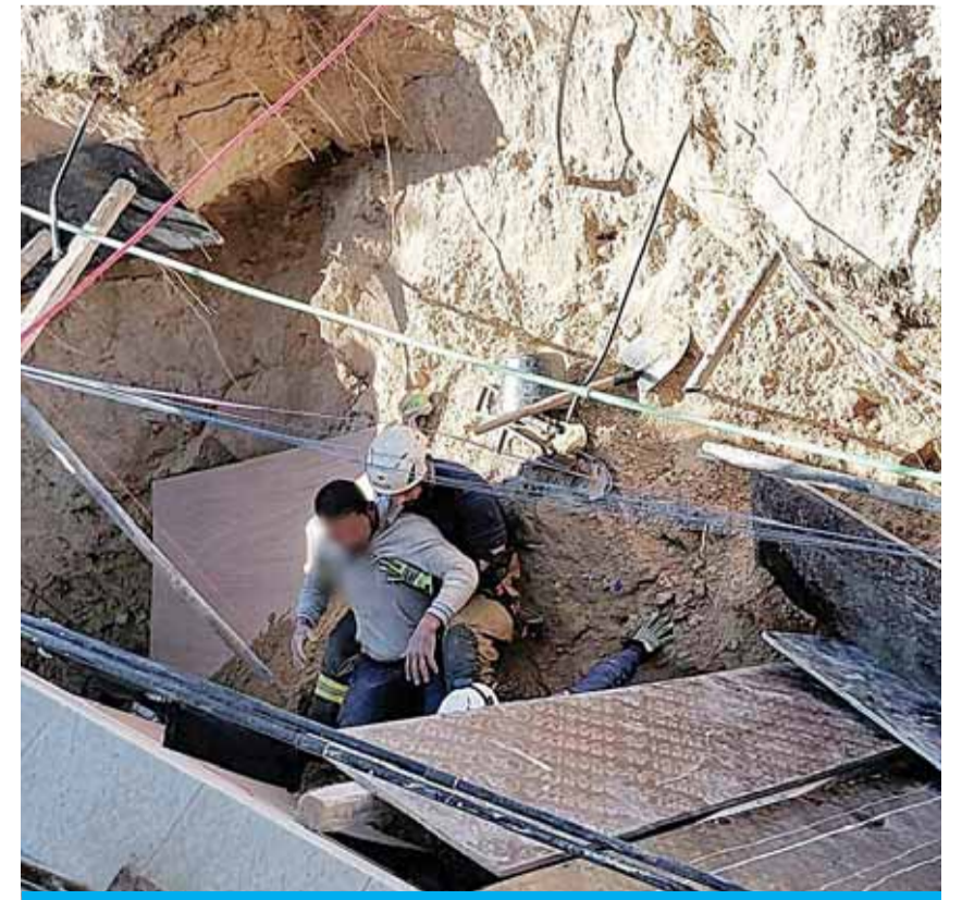
A fireman helps a worker after he became trapped following a landslide.
