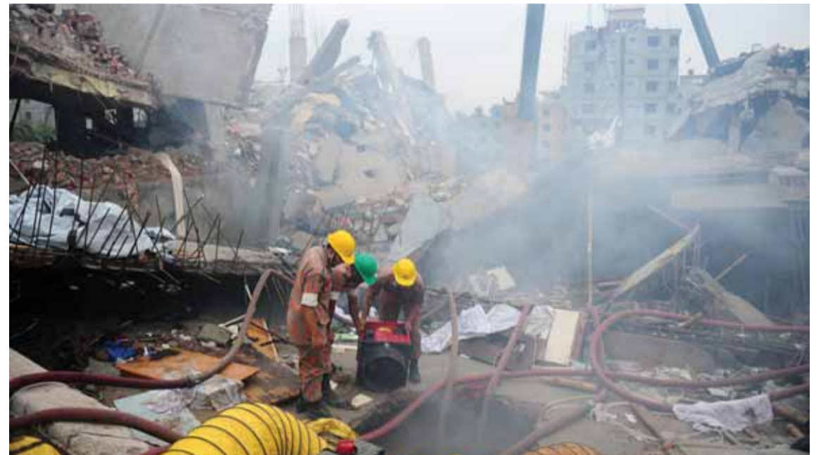
SAVAR: File photo shows, Bangladeshi firefighters try to control a blaze during a rescue attempt as Bangladeshi Army personnel begin the second phase of the rescue operation following the Rana Plaza building collapsed in Savar, on the outskirts of Dhaka. — AFP
