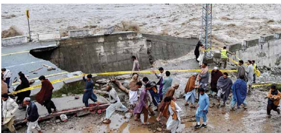
SWAT, Pakistan: People gather in front of a road damaged by floodwaters following heavy monsoon rains in Madian in the northern Swat Valley on Aug 27, 2022. — AFP
