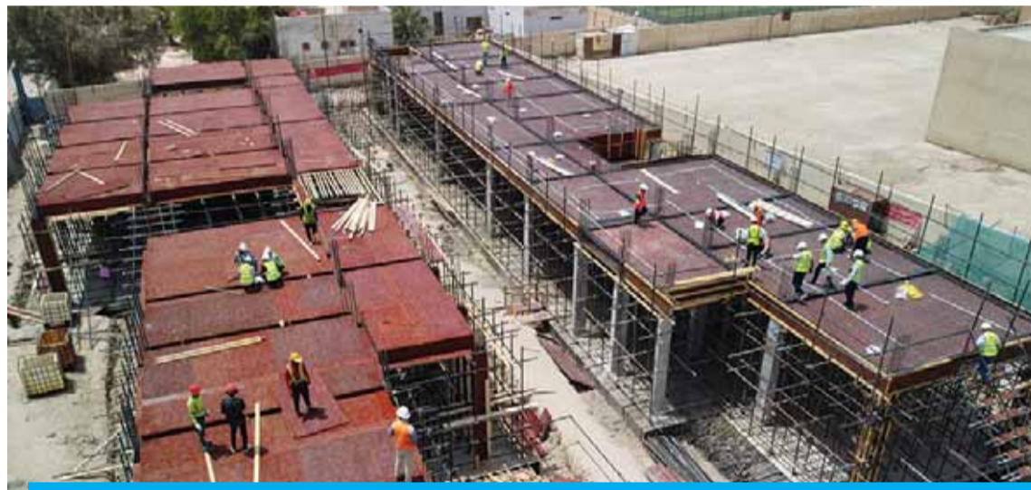
NASIRIYAH, Iraq: Laborers work on the construction site for a school, part of the Iraq-China "oil for construction" deal, in the Sumer neighborhood of Nasiriyah city, in Iraq's southern Dhi Qar province, on July 20, 2022. — AFP
