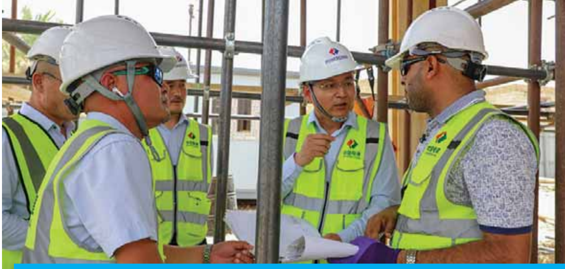
NASIRIYAH, Iraq: Supervisors talk at the construction site for a school, part of the Iraq-China "oil for construction" deal, in the Sumer neighborhood of Nasiriyah city, in Iraq's southern Dhi Qar province. — AFP
