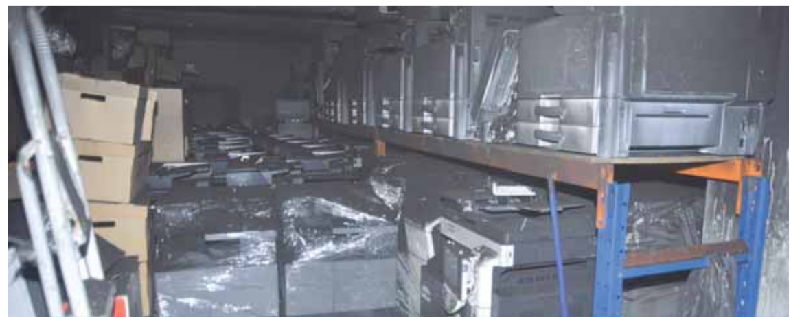
Charred goods are seen in a Jabriya basement.
