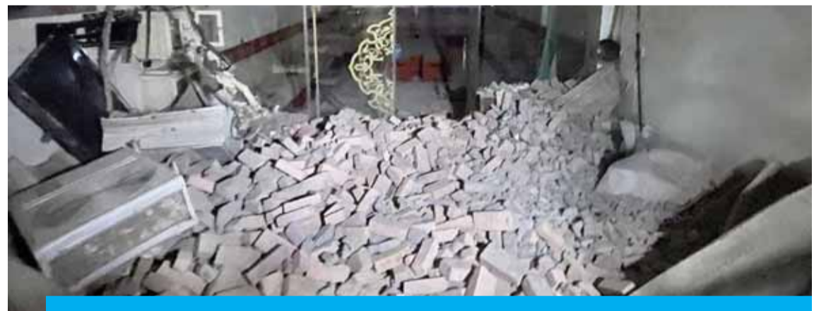
KUWAIT: The collapsed housefront of a building in Oyoum.
