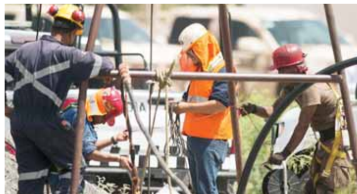
AGUJITA, Mexico: Rescue personnel work in the flooded coal mine where 10 miners have been trapped since Wednesday after a landslide, in the community of Agujita, Municipality of Sabinas, Coahuila State, Mexico. — AFP
