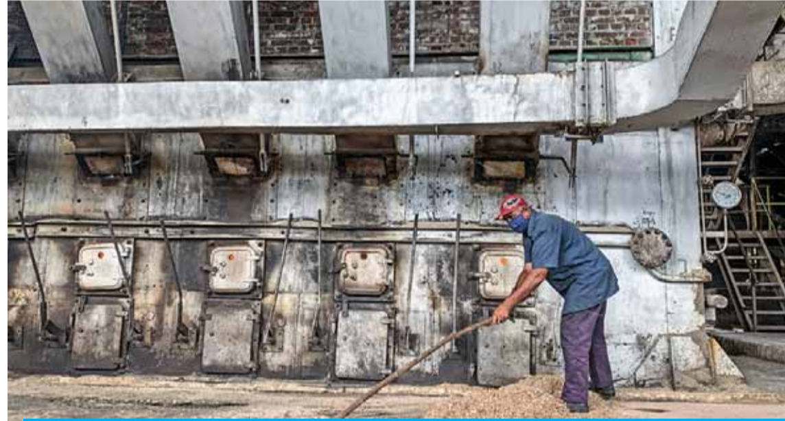
AGUADA DE PASAJEROS, Cuba: An operator controls the temperature of the furnaces that produce steam for electricity at the Antonio Sanchez Sugar Mill, in the town of Aguada de Pasajeros, Cienfuegos province, Cuba on March 17, 2022. — AFP
