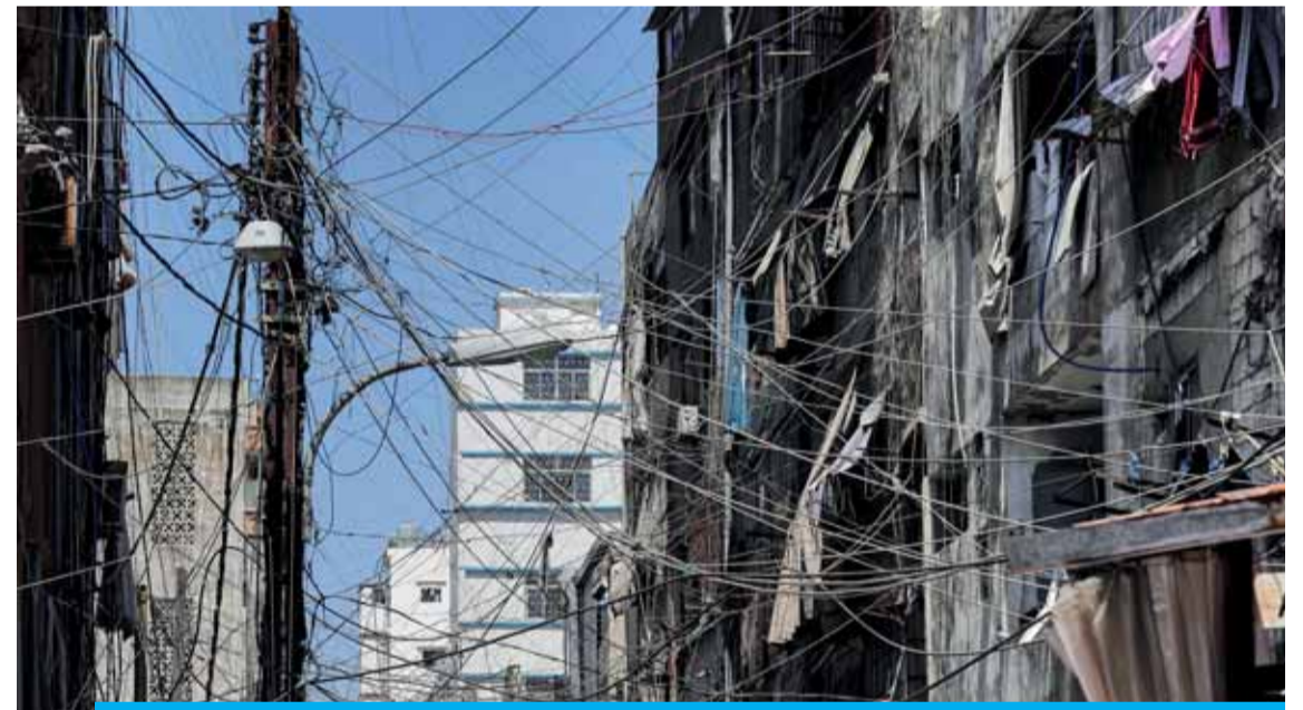
BEIRUT: Photo shows a view of a mesh of raised electricity lines along a street in a suburb of Lebanon's capital Beirut. — AFP
