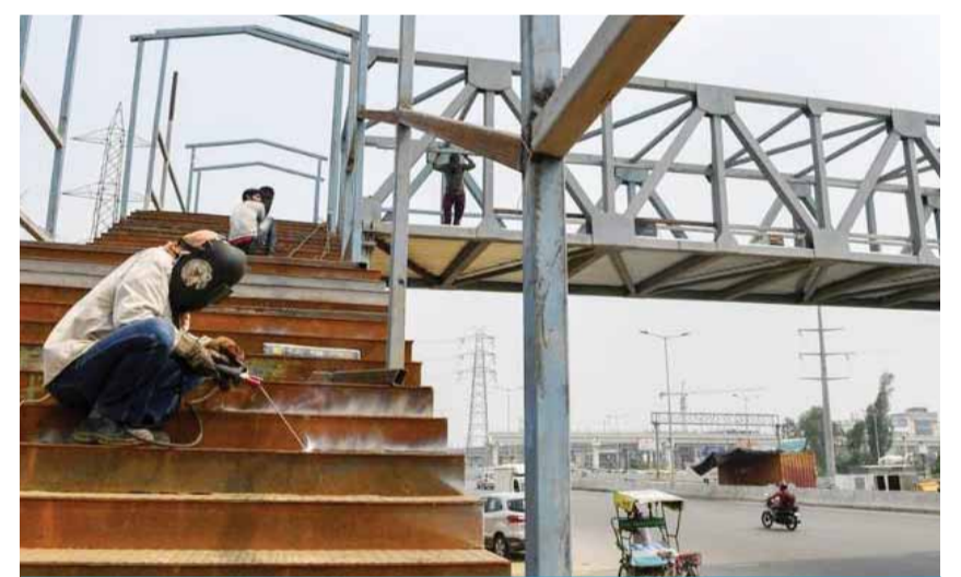
GHAZIABAD: Workers build a bridge in Ghaziabad, India. The Asian Development Bank has cut its growth forecast for developing Asia. —CAFP
