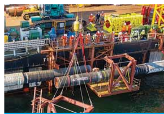
This undated handout picture taken in September 2021 and provided by Nord Stream 2 AG, shows specialists on the lay-barge Fortuna performing an above water tie-in during the final stage of Nord Stream 2 pipeline construction in the Baltic Sea. —AFP
