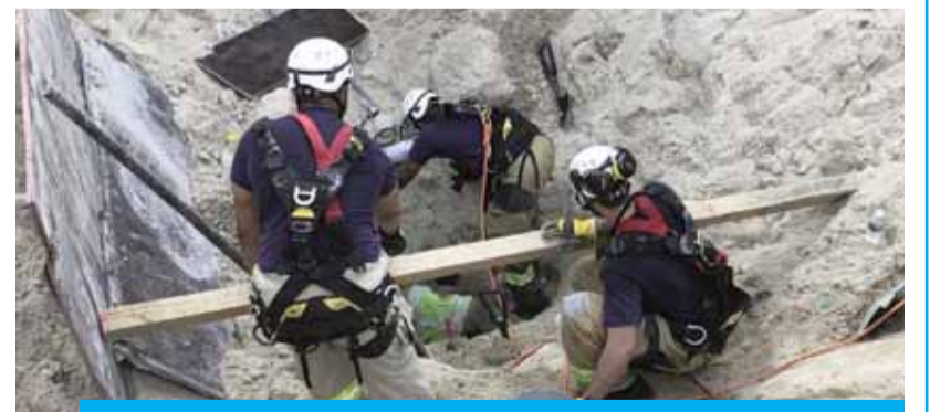
KUWAIT: Rescuers work to extract three workers buried in sand at the Kuwait airport construction site yesterday. — KUNA
