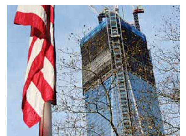
NEW YORK: This file photo shows the One World Trade Center tower under construction in New York. It is the skyscraper that replaced the Twin Towers in New York's skyline. —AFP
