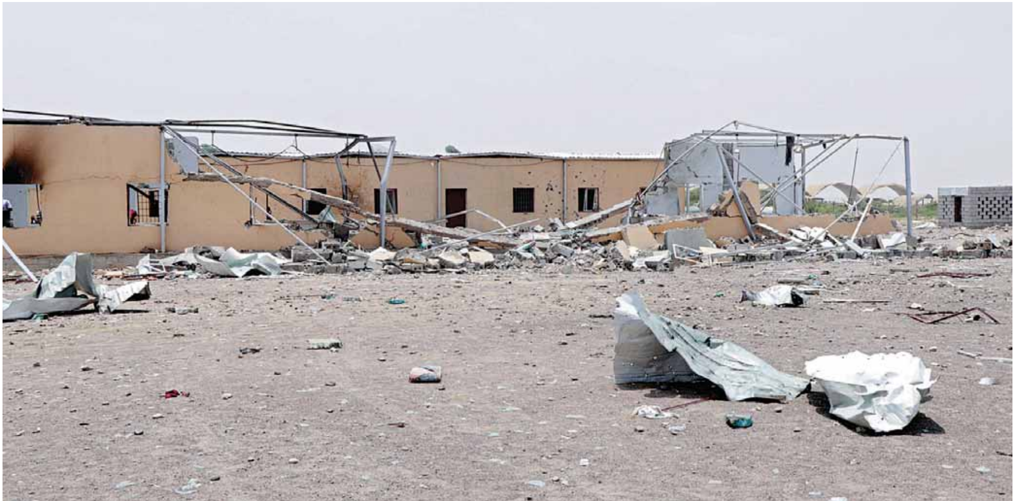
ADEN: Photo shows the damage at the Al-Anad airbase, some 60 kilometers north of Yemen's second city Aden, after it was reportedly targeted by Houthi rebels. —AFP
