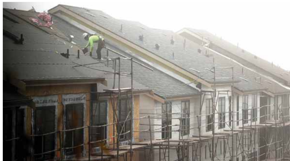
SOUTH SAN FRANCISCO: A worker stands on the roof of a new home under construction in South San Francisco, California.— AFP
