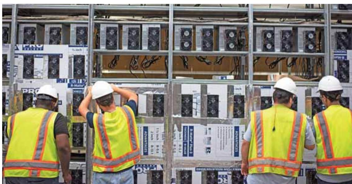
ROCKDALE, US: Workers install a new row of Bitcoin mining machines at the Whinstone US Bitcoin mining facility in Rockdale, Texas. —AFP
