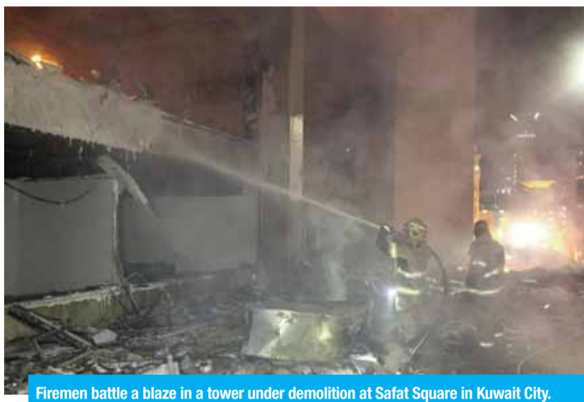
Firemen battle a blaze in a tower under demolition at Safat Square in Kuwait City.
