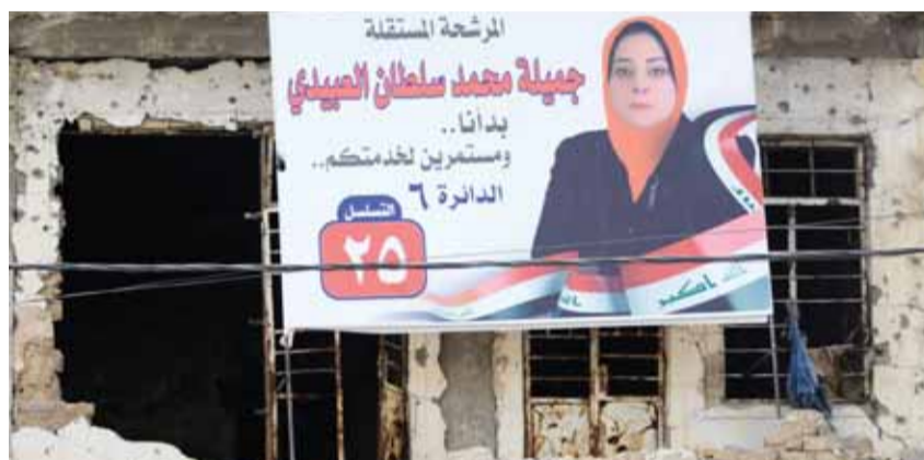
MOSUL: An electoral banner hangs on the facade of a damaged building in Iraq's second city of Mosul, in the northern Nineveh province yesterday ahead of the upcoming parliamentary elections. — AFP
