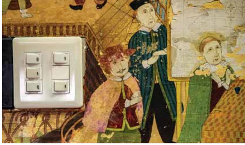
This picture shows light switches (L) next to ageing decorations on a wall of Taiyoshi Hyakuban.
