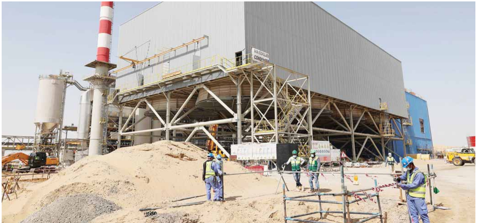
SHARJAH: Workers are pictured next to a waste management facility under construction at the Bee'ah company in the Gulf emirate of Sharjah. — AFP
