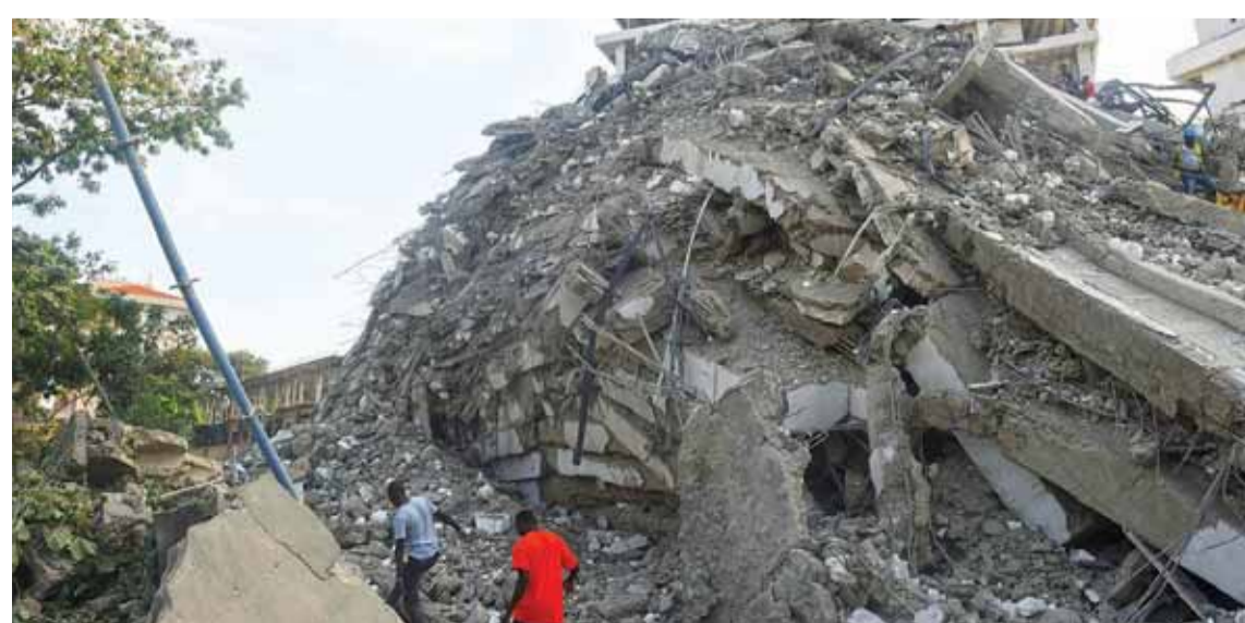
LAGOS: People walk to rescue workers from the rubble of a 21-storey building under construction that collapsed at Ikoyi district of Lagos. — AFP
