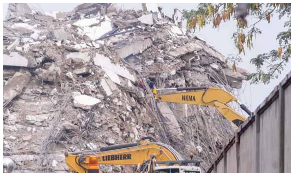
IKOYI, Nigeria: Rescue workers search for survivors still trapped under the rubble at the site of the collapsed 21-storey building in Ikoyi, Lagos yesterday. —AFP
