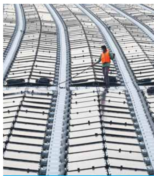
SINGAPORE: A worker pulling a cable along a floating solar power farm at sea, off Singapore's northern coast just across the Malaysian state of Johor. — AFP
