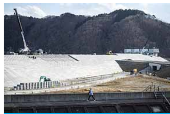
MIYAKO, Japan: In this picture a woman walks along an old sea wall as construction workers (behind) build a newer and higher one in the Taro district of Miyako, Iwate Prefecture. —AFP
