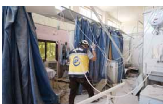
AFRIN, Syria: A member of Syria's Civil Defense service (White Helmets) inspects the damage yesterday in one of the rooms of the Al-Shifaa hospital, a day after it was hit by artillery shells in the rebel-held northern Syrian city of Afrin, reportedly fired by pro-regime forces, killing at least 18 people, and wounding more than 23, according to a war monitor. —AFP
