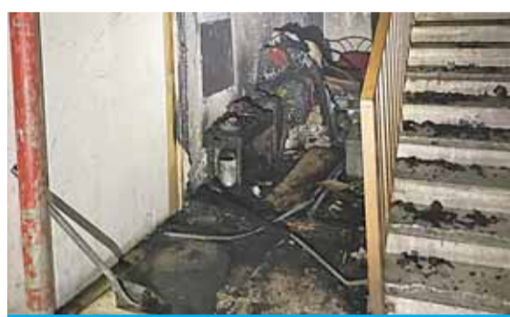
Damage left by a fire inside the Jahra building.
