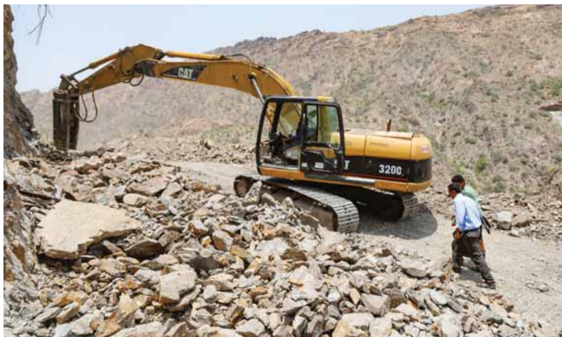
TAEZ, Yemen: This picture taken in the mountains near Yemen's third city of Ta'ez, shows the construction of a road that will serve as a lifeline between Ta'ez, besieged by Houthi rebels, and the southern city of Aden, the internationally recognized government's temporary capital. — AFP
