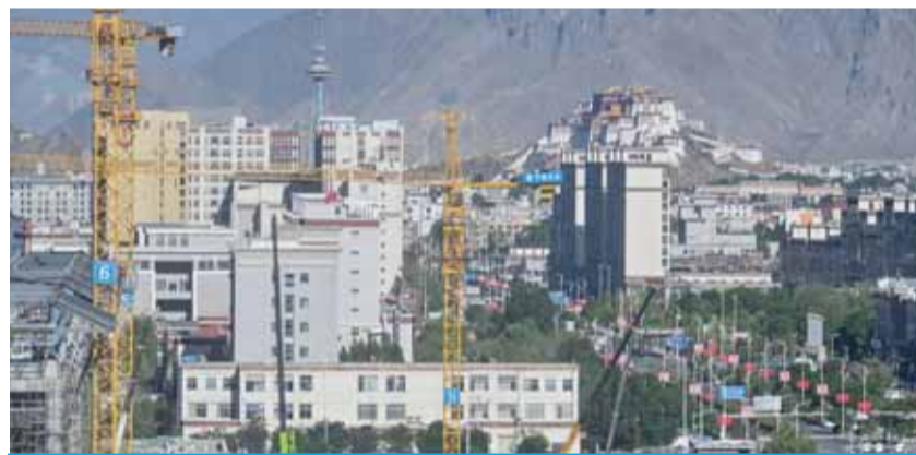
This photo taken on June 3, 2021 shows a general view of new building sites under construction in the regional capital Lhasa in China's Tibet Autonomous Region. —AFP
