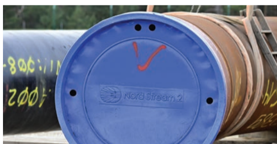
LUBMIN, Germany: A pipe is seen at the construction site of the so-called Nord Stream 2 gas pipeline in Lubmin, northeastern Germany. — AFP
