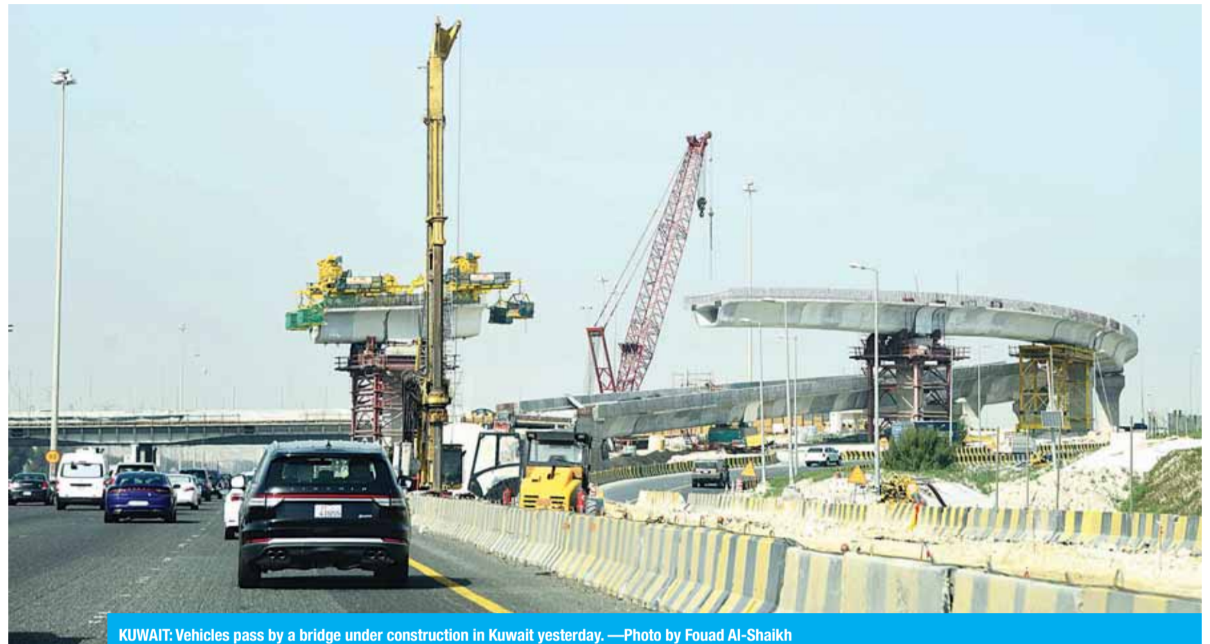
KUWAIT: Vehicles pass by a bridge under construction in Kuwait yesterday. —Photo by Fouad Al-Shaikh
