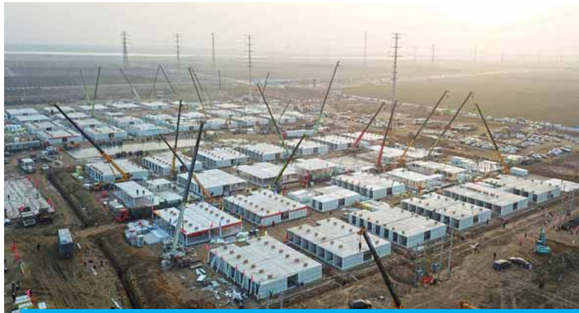
SHIJIAZHUANG, China: This aerial photo shows the under-construction centralized quarantine facilities, where people at risk of contracting the COVID-19 are to be taken into quarantine.— AFP
